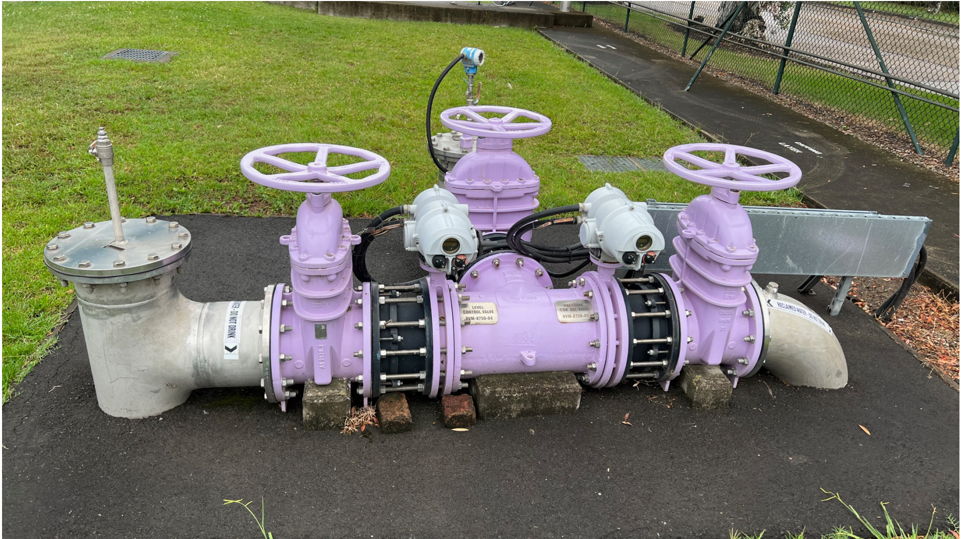
Figure 1. Typical example of clearly labelled, coloured and signed recycled water infrastructure (Rosehill).
