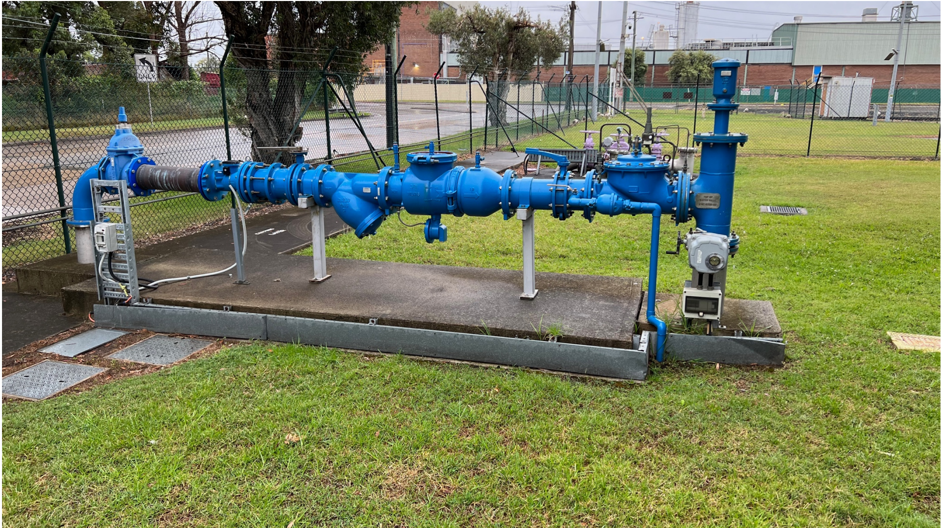
Figure 2. Typical example of clearly coloured and potable water backup infrastructure with testable backflow prevention device (Rosehill).
