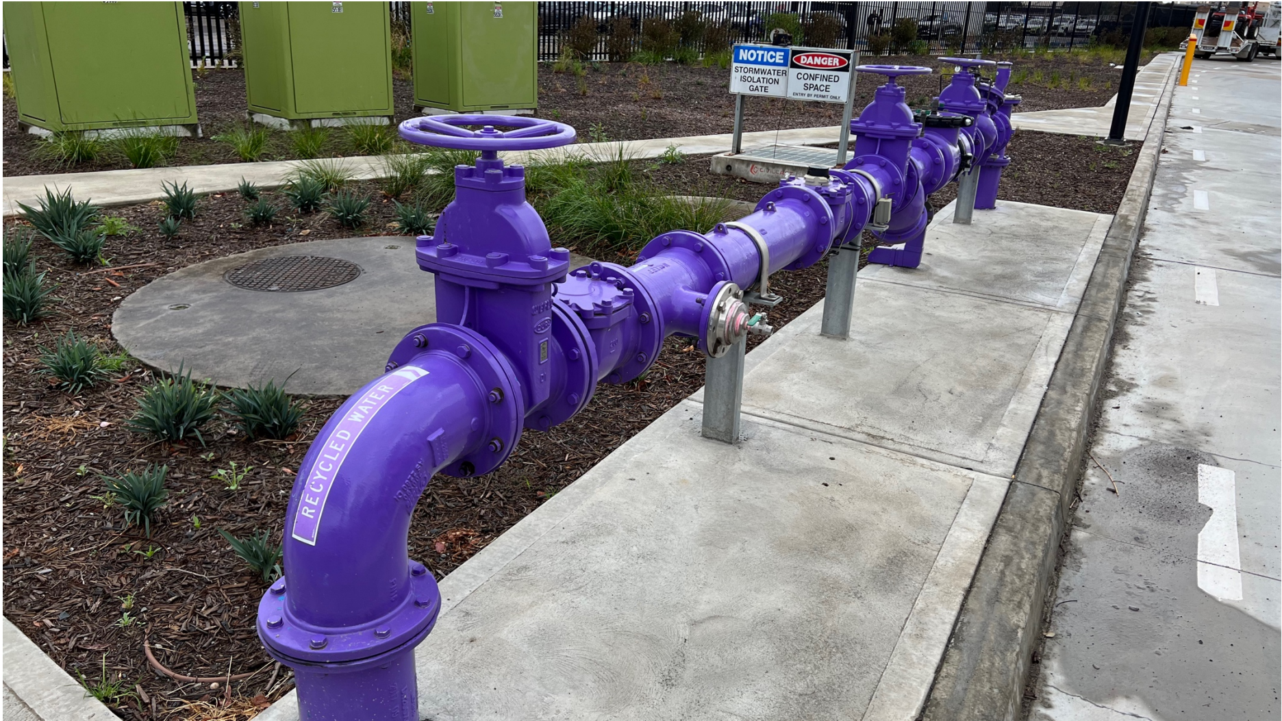
Figure 6. New connection to Equinix customer with appropriate parts, fittings, labelling and signage.
