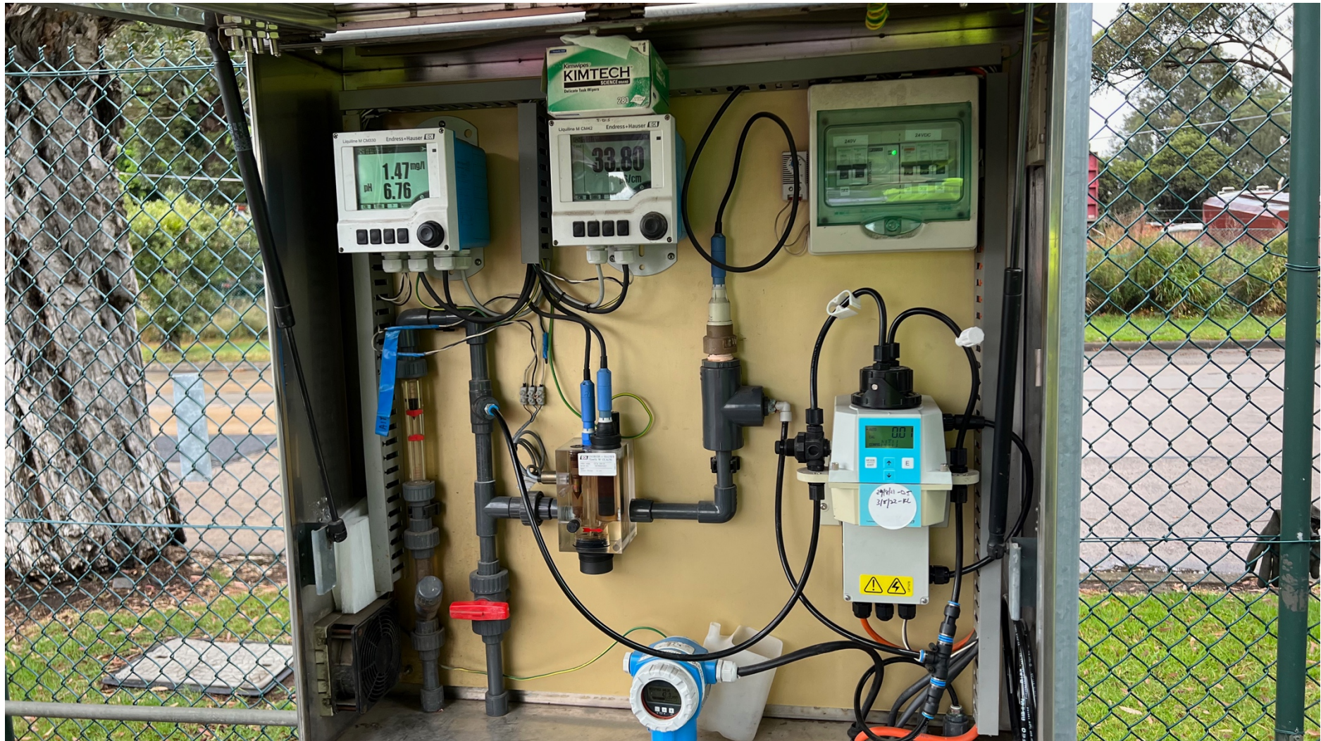
Figure 3. Typical example of fully functional wet rack, in good condition (Rosehill).
