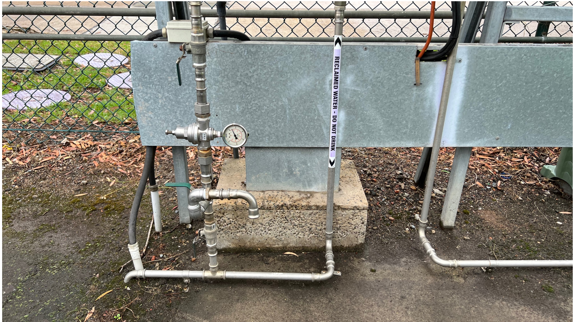
Figure 4. Typical example of appropriate water sampling tap, in good condition (Rosehill).
