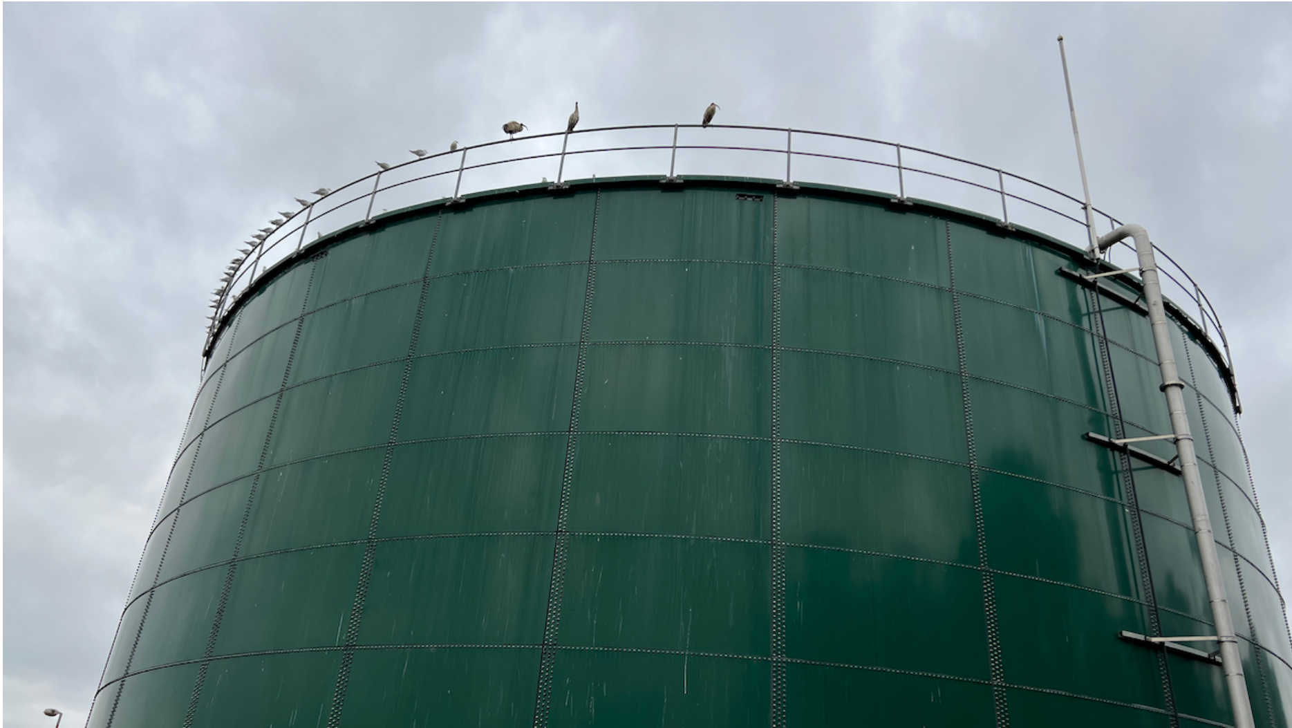
Figure 5. Potable water top fill line into treated water storage tank (Rosehill).
