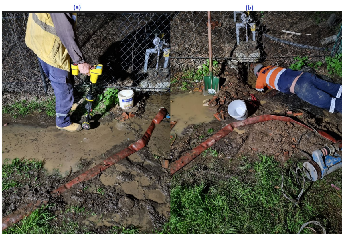
Figure 6: Photographs of the pipe leak scene at CSR Monier with gas monitoring (a) and during pipe fixing (b).
